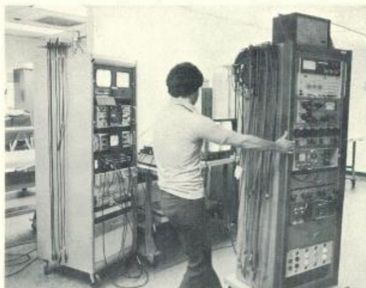
Test bays are mobile so that movement of disassembled gear is minimized
